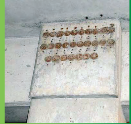
Evidence of corrosion at post-tensioning grout pockets
