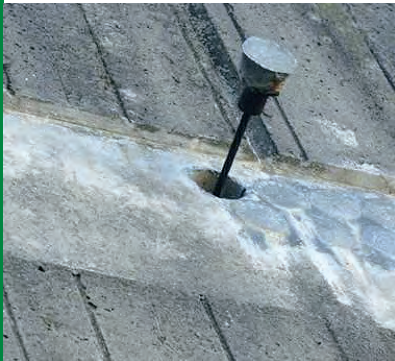
Post-tensioned tendon failures can erupt from the structure
