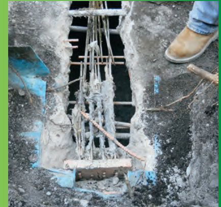
Failure of paper wrapped, button headed wire post-tensioning system
