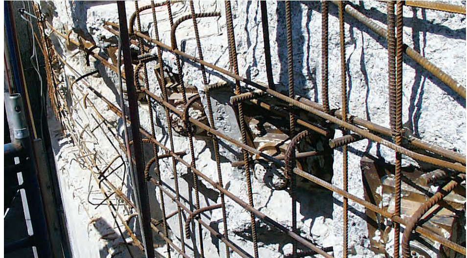
Post-tensioned nuclear containment building required concrete repairs and FRP strengthening
