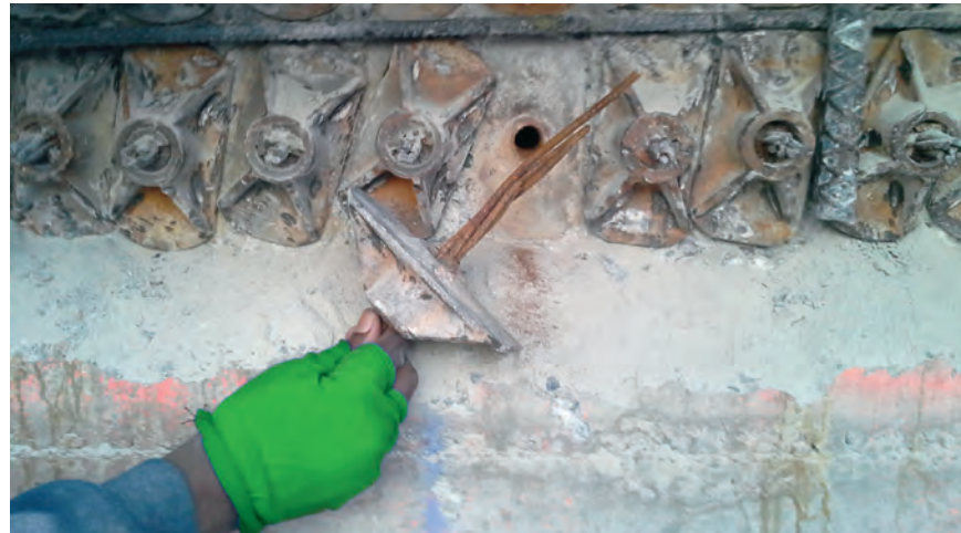
Corrosion of post-tensioned strand adjacent to an anchor plate
