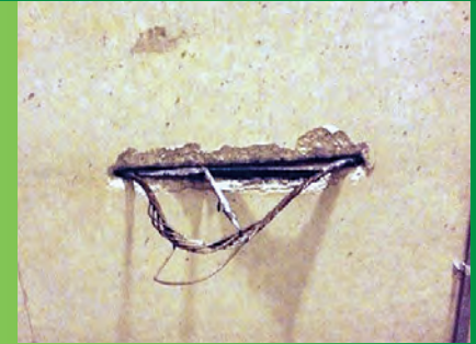
Eruption of broken unbonded post-tensioned tendon
